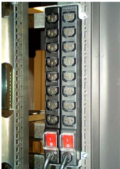
Figure 6. Double-mounted power strips.
