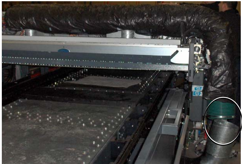
Figure 8-2 Fume Extraction Duct
