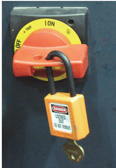
Figure 1-2 Lock-out of the Main Power Switch
