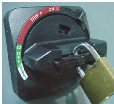
Figure 1-9 UV Main Isolator locked in the OFF position
