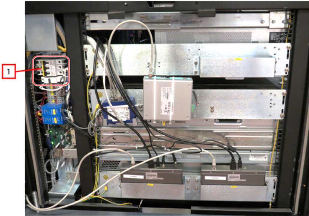
1 24V circuit breakers
