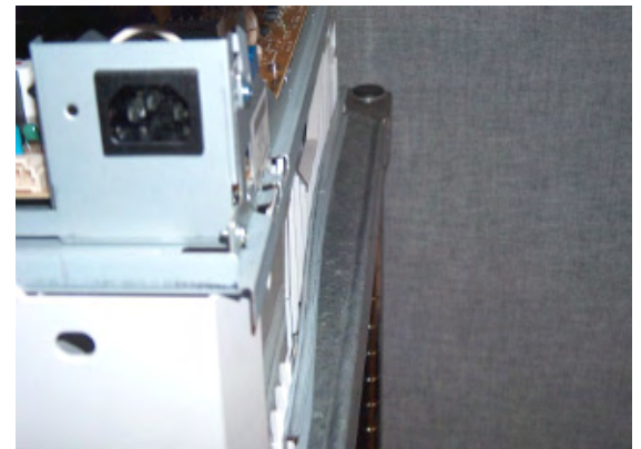
The rear cover is removed, showing that the crossbar on the chassis is bowing inward more than normal
